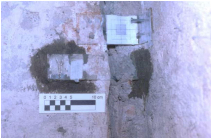
Telltale crack monitoring device (NHCP-HPD photo collection)
