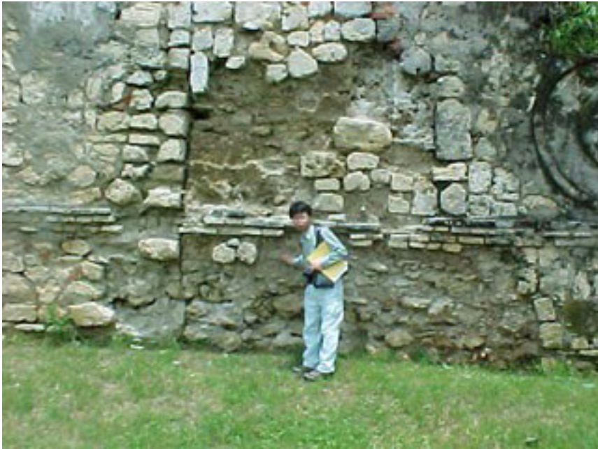
Dr. Hanazato inspecting damaged wall of Paoay Church (NHCP-HPD photo collection)
